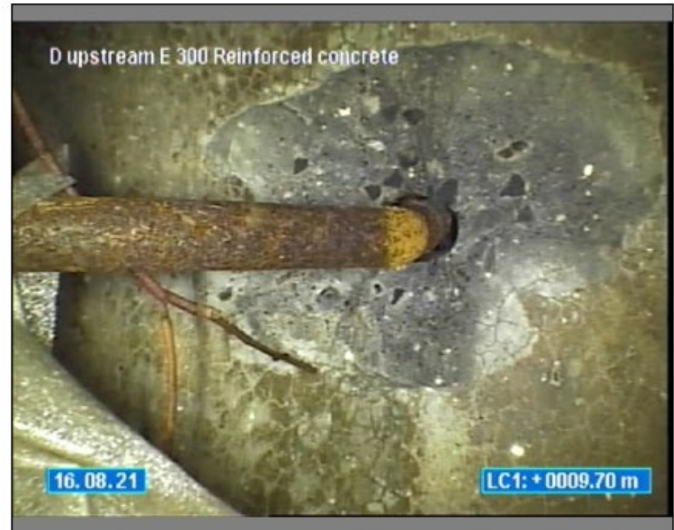
Photo: 0_16082021_121754_E_4_4A.JPG 9.7m, Obstruction, an object is intruding through the wall , reduction in cross sectional area: 5-20%, STEEL REBAR, at 12 o'clock
