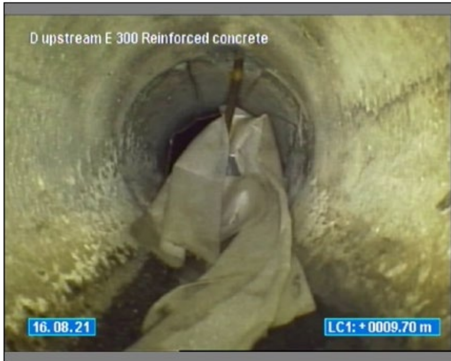
Photo: 0_16082021_121808_E_4_4A.JPG 9.7m, Obstruction, an object is intruding through the wall , reduction in cross sectional area: 5-20%, STEEL REBAR, at 12 o'clock
